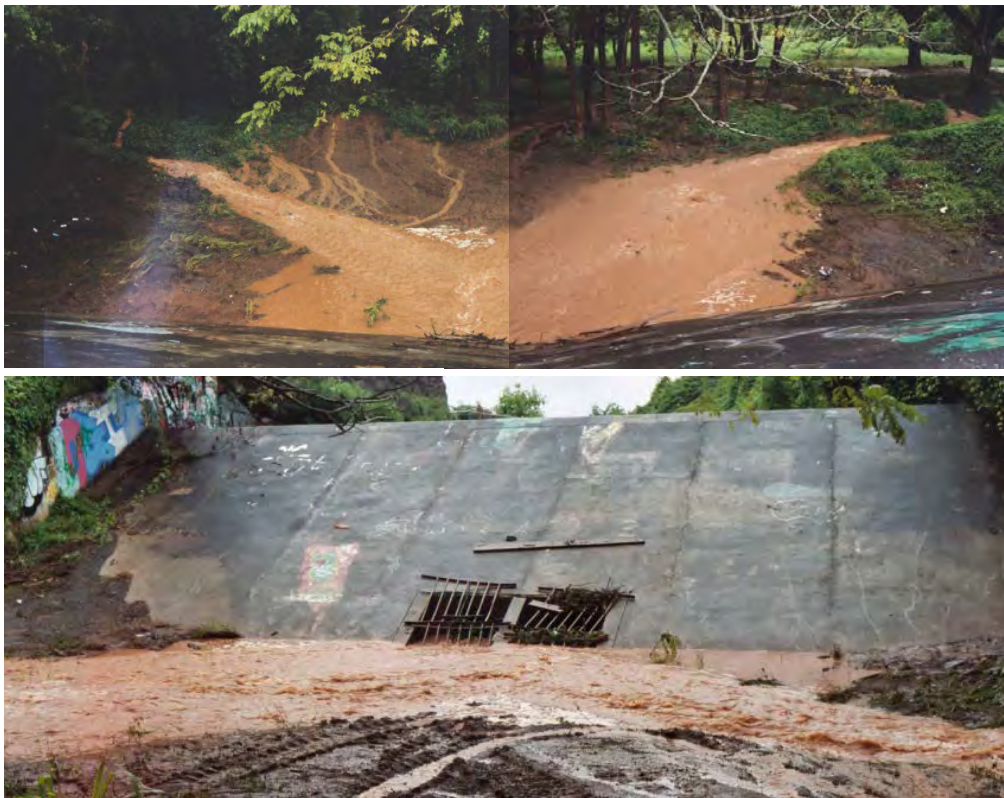
Figure 26. Top: Looking down the inside Keopu dam face as muddy water pours through the two erosional channels cut through the internal raised berm. Bottom: Inside the basin looking at the back of the dam face with the muddy water flowing into the two flow control structures beneath the dam.
