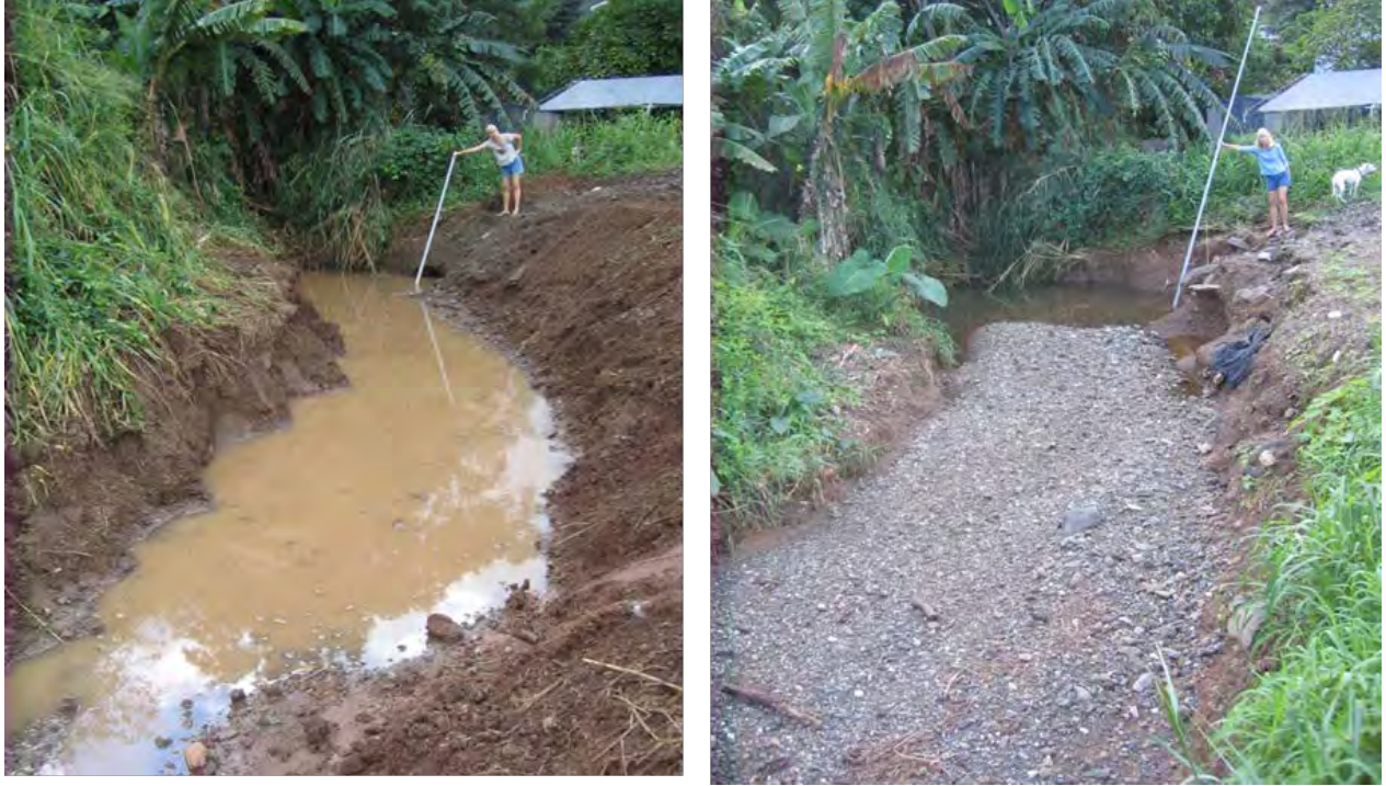
Figure 25. Before (left) and after(right) sediment from a City storm drain filled this swale during a single storm. The staff is a 16-foot survey rod.
