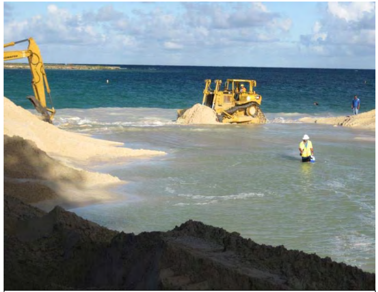
Figure 29 The City uses heavy equipment to open the stream mouth about nine times per year.
