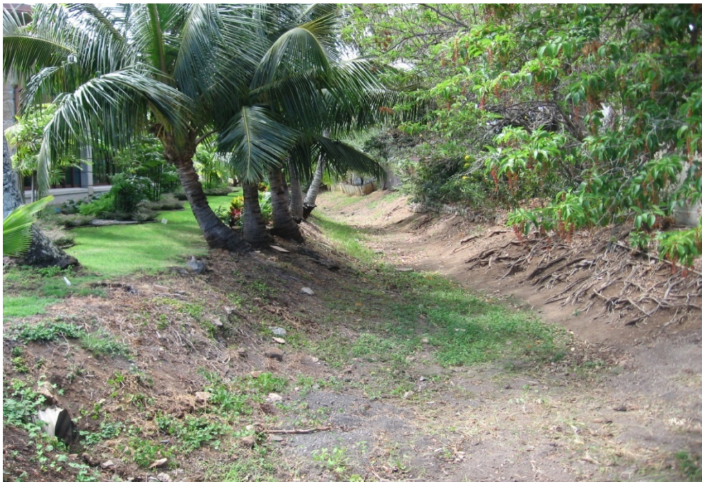
Photo 1-22 Kamahele earthen ditch looking southwest from Keolu Drive. Note scouring of embankment, road debris accumulation in the ditch, and church drainpipe outlet .
