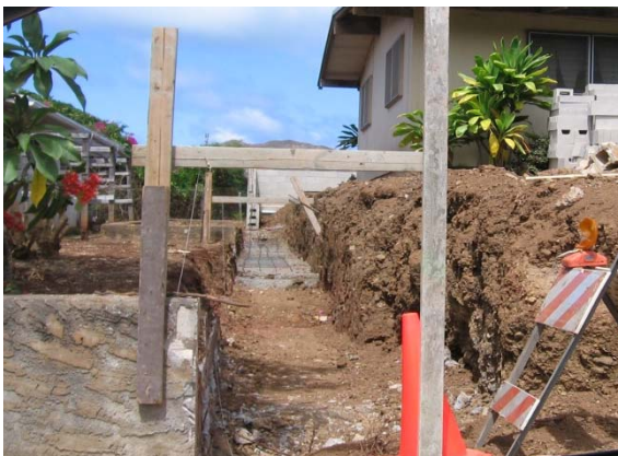
Photo 1-57 Residential construction site on Keolu Drive without BMPs. Pollutant source area for storm water runoff into WKIP 42 drainage system.
