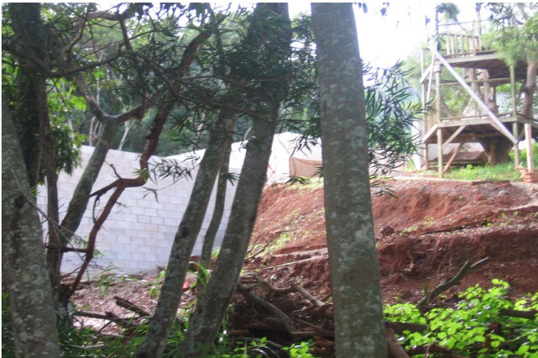
Photo 2-2 Construction site along Old K-Hwy. Structural BMPs were not observed on site.
