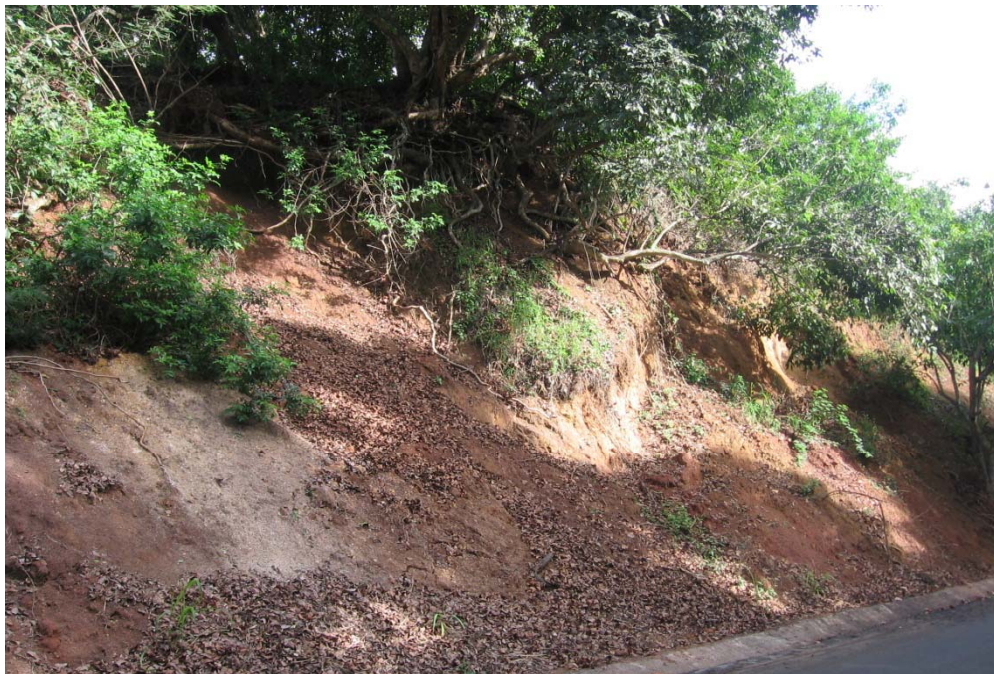
Photo 2-4 Steep, barren embankments along Old K-Hwy are common.
