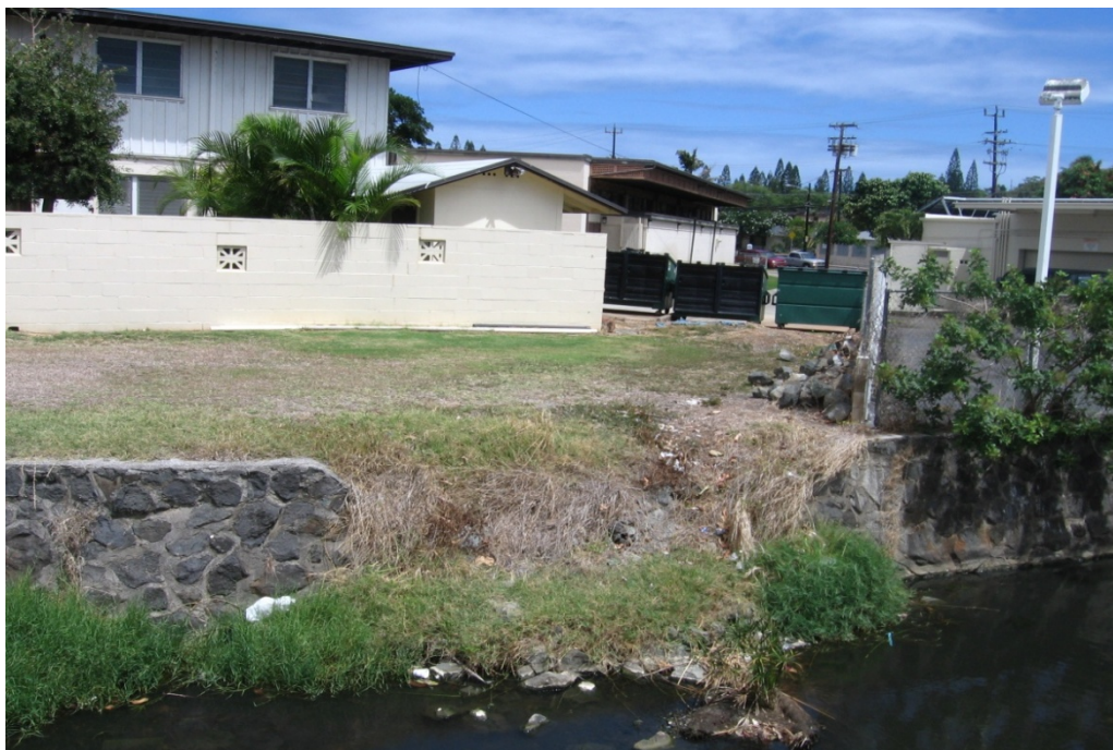
Photo 1-38 Dilapidated wall on north side of Hele Channel near Keolu Drive.
