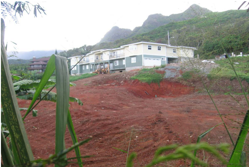
Photo 2-1 Construction site along Old K-Hwy. Structural BMPs were not observed on site. Photo taken from K-Hwy.
