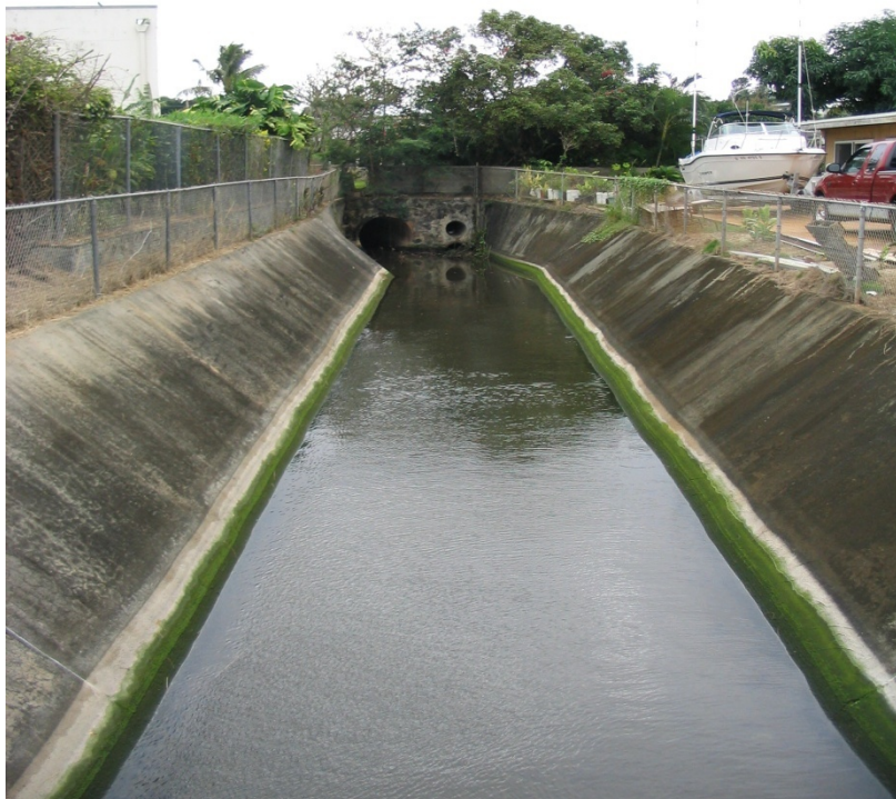
Photo 1-4 Photo taken from Alahaki Street Bridge looking northeast (upstream) of Interceptor Ditch #1. Note corner of movie theater from Enchanted Lake Shopping Center, relief drain and pipe from Keolu Drive.
