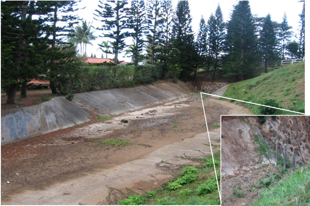
Photo 1-55 Concrete lined silt off of Old Kalaniana'ole Highway, which is part of WKIP 34 outlet discharging into Kapaa Silt Basin.
