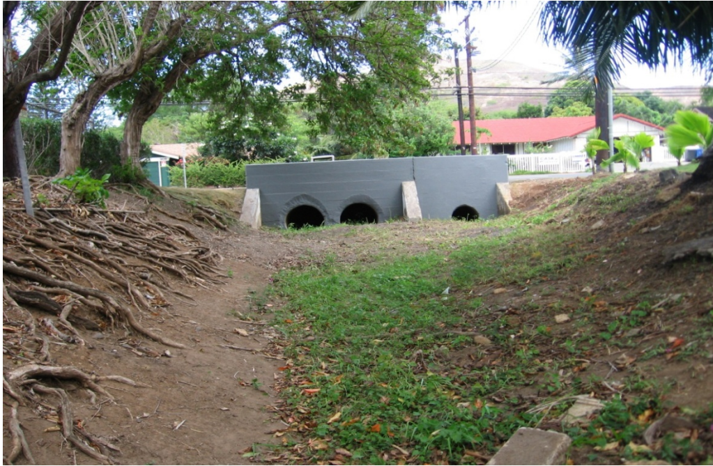
Photo 1-21 Kamahele Ditch looking northeast toward Keolu Drive. Recommended area for ditch excavation of deposited soils and bank stabilization (both sides) using vegetative riprap and/or mechanical revetment.
