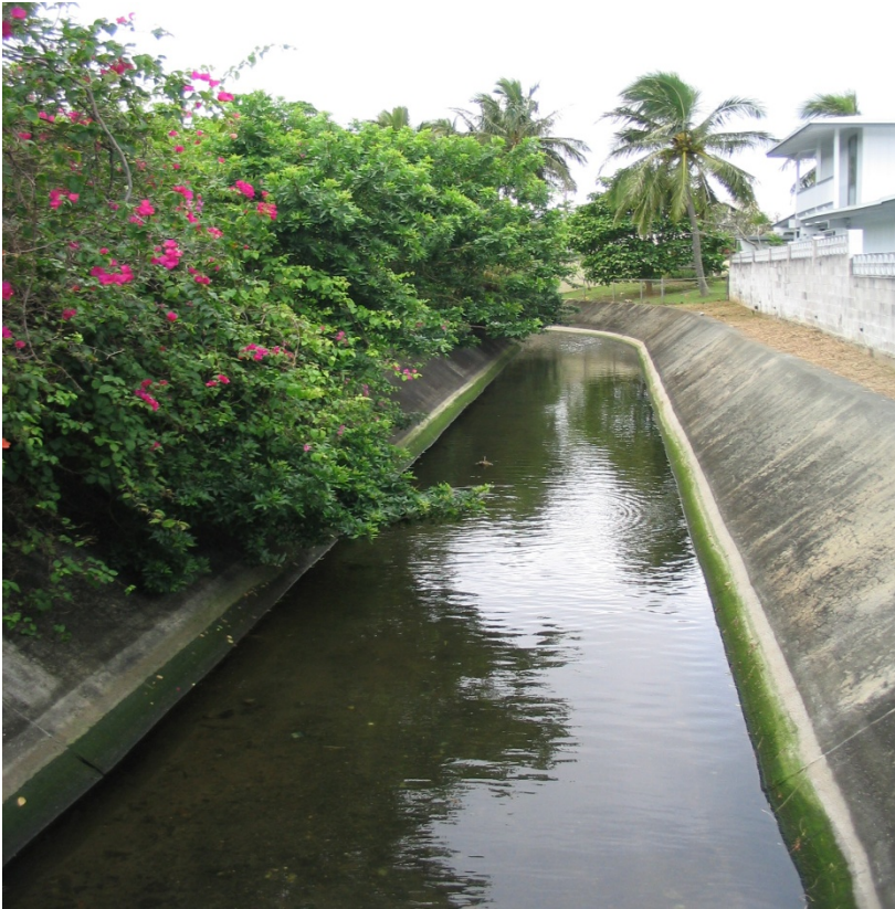
Photo 1-3 Photo taken from Alahaki Street Bridge looking northwest (downstream) of Interceptor Ditch #1.
