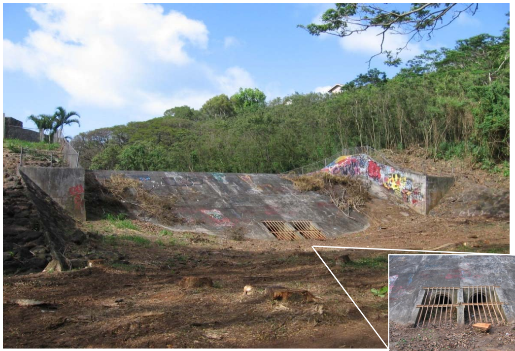
Photo 1-46 City debris control system at beginning of Keolu Lined Channel. Note recently cleared area with debris scattered. Grated inlet houses two 18-inch RCPs.
