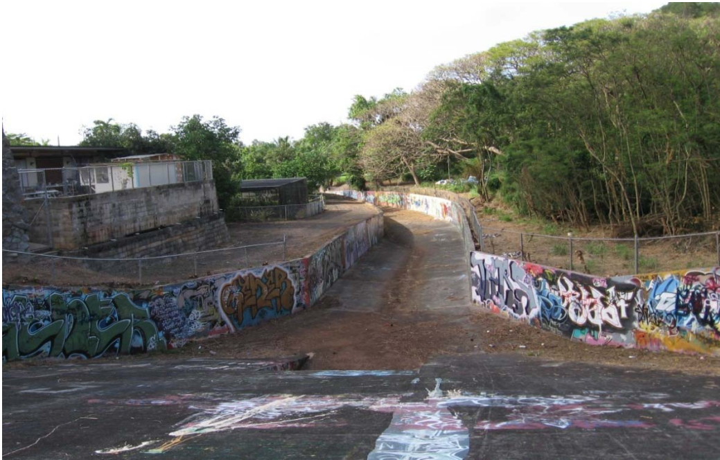
Photo 1-45 Keolu Lined Channel looking downstream (north) from on top of the City debris control system. Paint can debris is a common.
