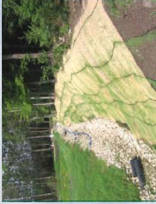
Vegetative swale, can be implemented to retain sediment and decrease velocity of stormwater runoff.
