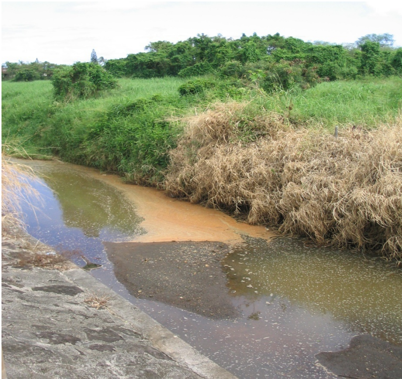
Photo 1-41 End of Keolu Lined Channel and beginning of unlined portion of channel. Note this area is typically stagnant, even during significant flows (see following photo) due to increased depth from scouring of unlined channel bottom.
