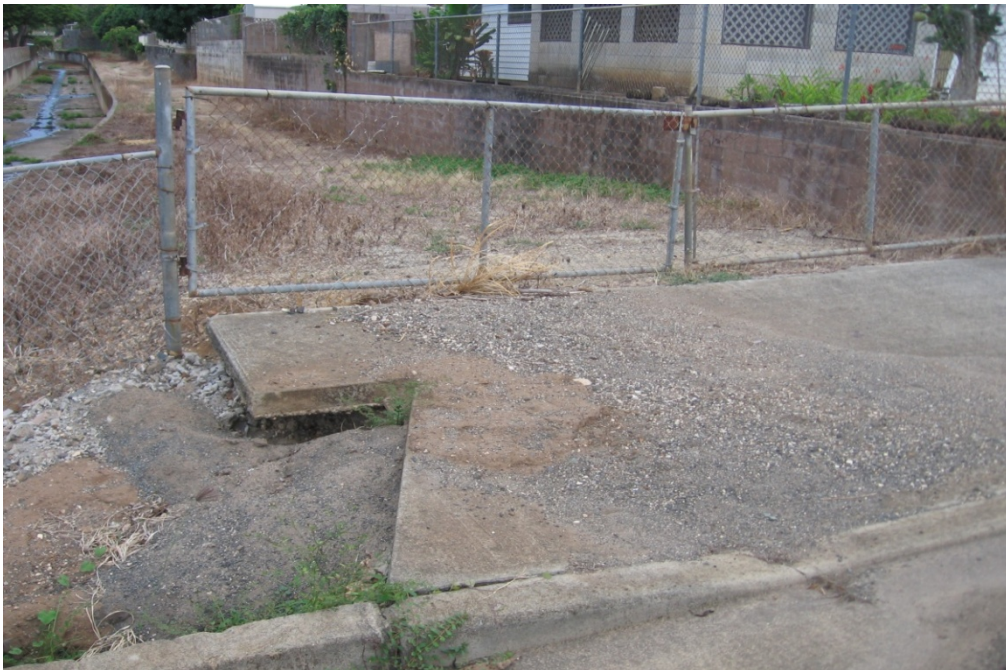
Photo 1-54 Erosion and sediment deposits at the end of Akumu Street. Note Keolu Lined Channel and City access easement in background.
