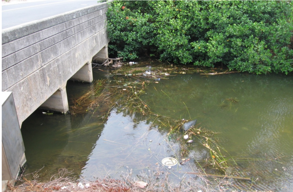
Photo 1-37 WKIP 10 drainage area Akumu Street Bridge. Potential location for vegetation screening bars.
