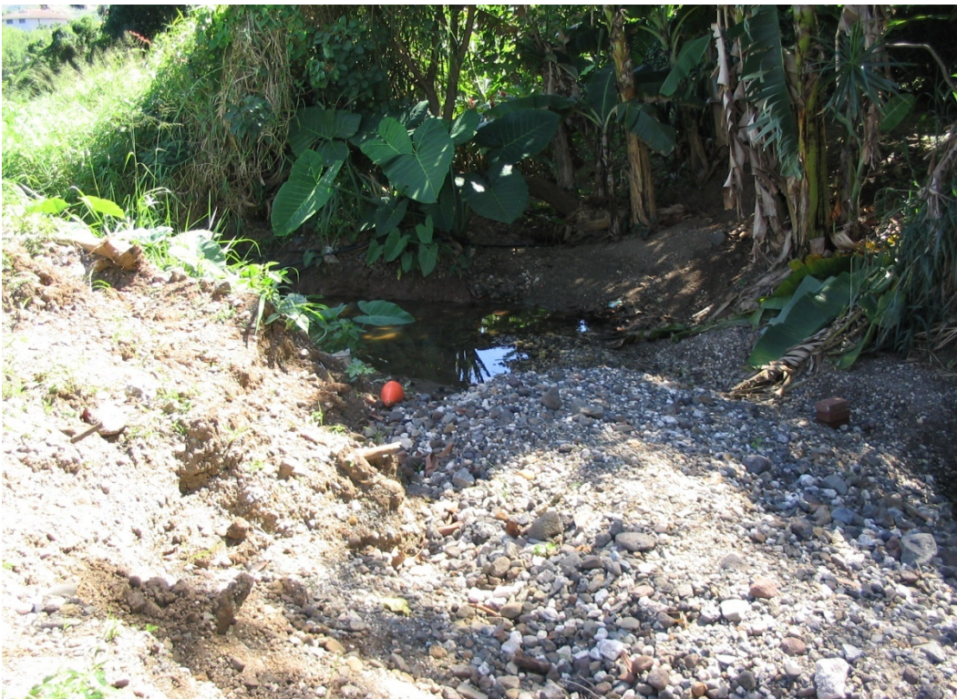
Photo 1-52 WKIP 43 outlet buried by sediment and debris.
