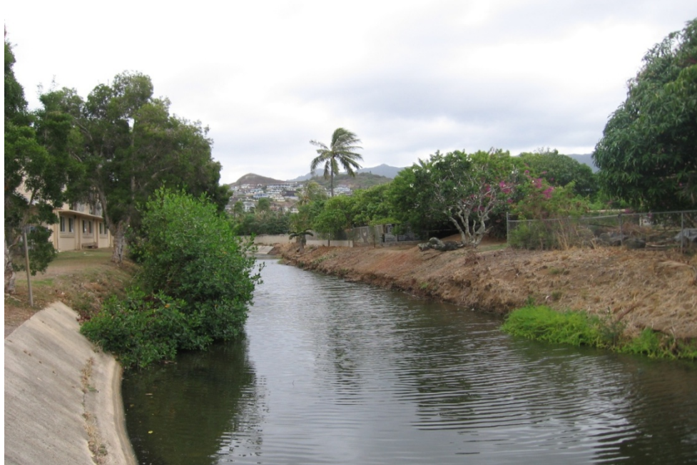
Photo 1-25 WKIP 10 Hele Drainage Channel looking south from Kamahale Ditch junction. Note erosion of unlined channel bank. Recommended bank stabilization area using vegetative riprap and/or mechanical revetment.
