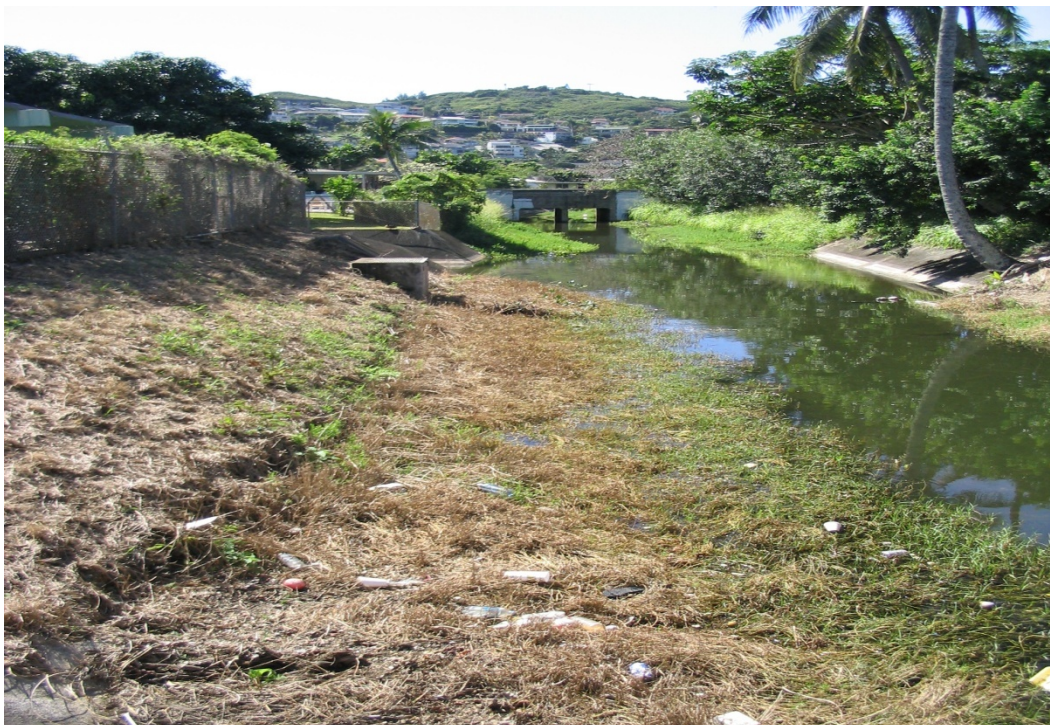
Photo 1-2 Alahaki Ditch looking upstream toward Kahili Street Bridge. Note Interceptor Ditch #1 junction and excessive dead vegetation from spraying.
