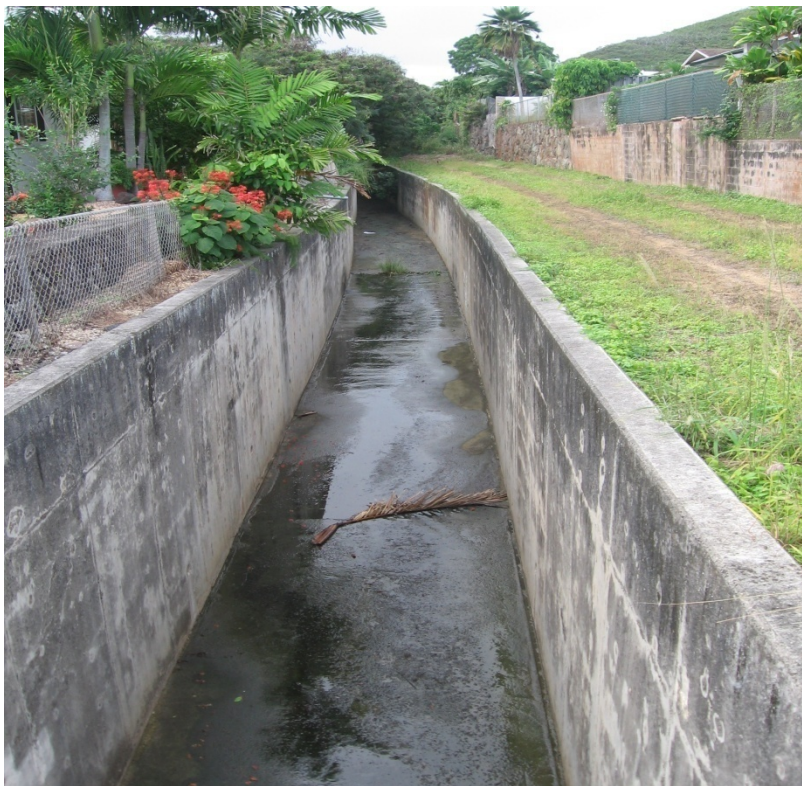
Photo 1-10 Akipola Lined Channel looking upstream. Note: City and County maintenance easement extends to beginning of channel.
