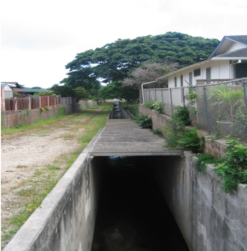
Photo 1-9 Akipola Lined Channel looking downstream. Note: concrete covering over this section of the channel helps reduce green waste buildup in the channel.
