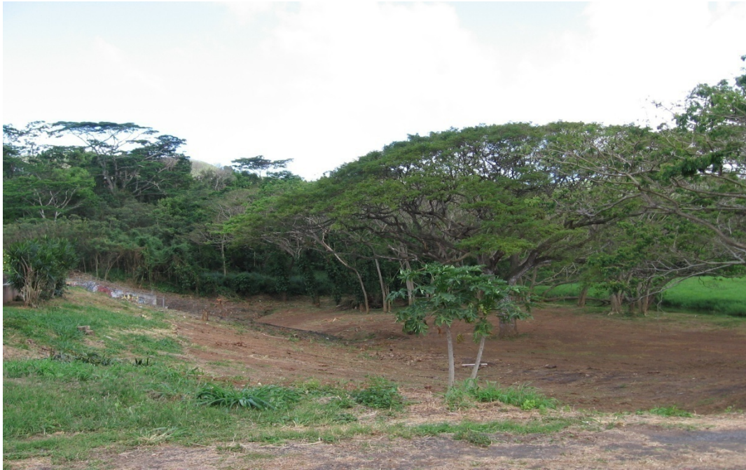
Photo 1-47 Cleared area between City debris control structure (left side of photo) and Kapaa Silt Basin (grass on right side of photo).
