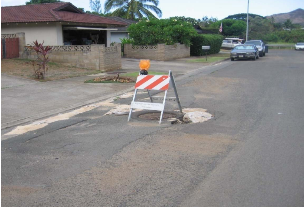
Photo 1-53 Storm drain manhole on Akumu Street is frequently popped during storm events due to back pressure from WKIP 43 outlet blockage and 90-degree alignment bend at this junction.
