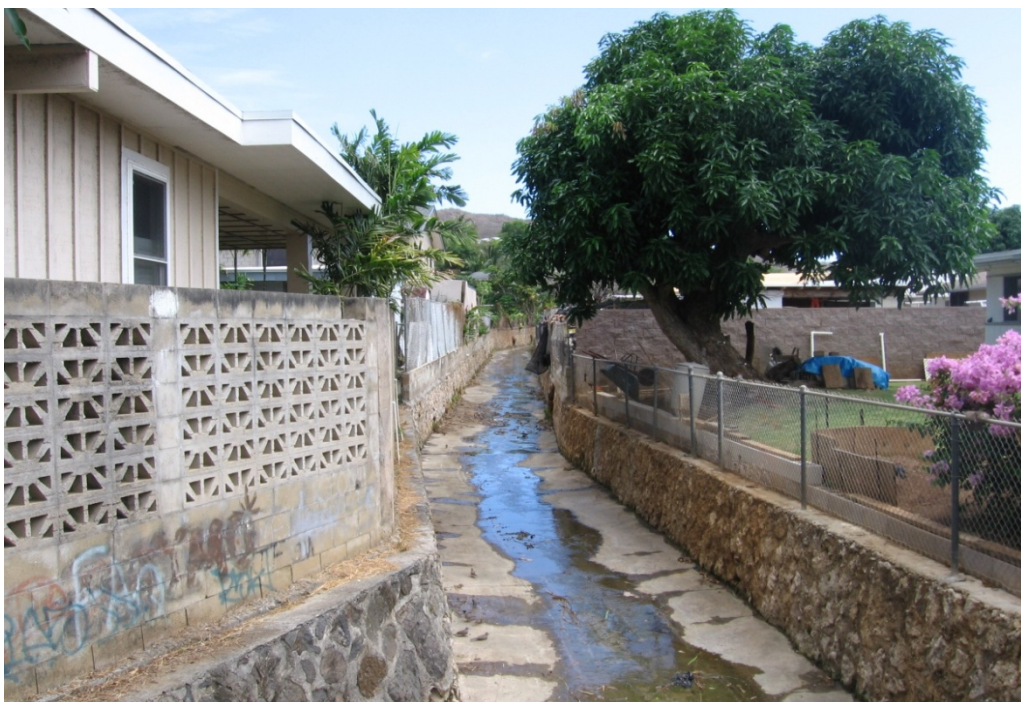
Photo 1-31 Hele Drainage Channel looking east from 6 th parcel from Liku Street Bridge. Two RCPs (24 and 36-inch) come in from Loho Street here.
