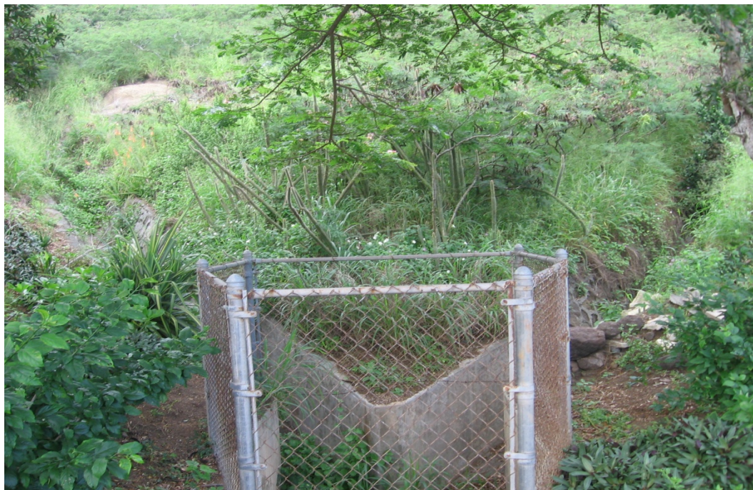
Photo 1-14 showing lined drainage ditch collection system from the hill behind Akiohala Place.
