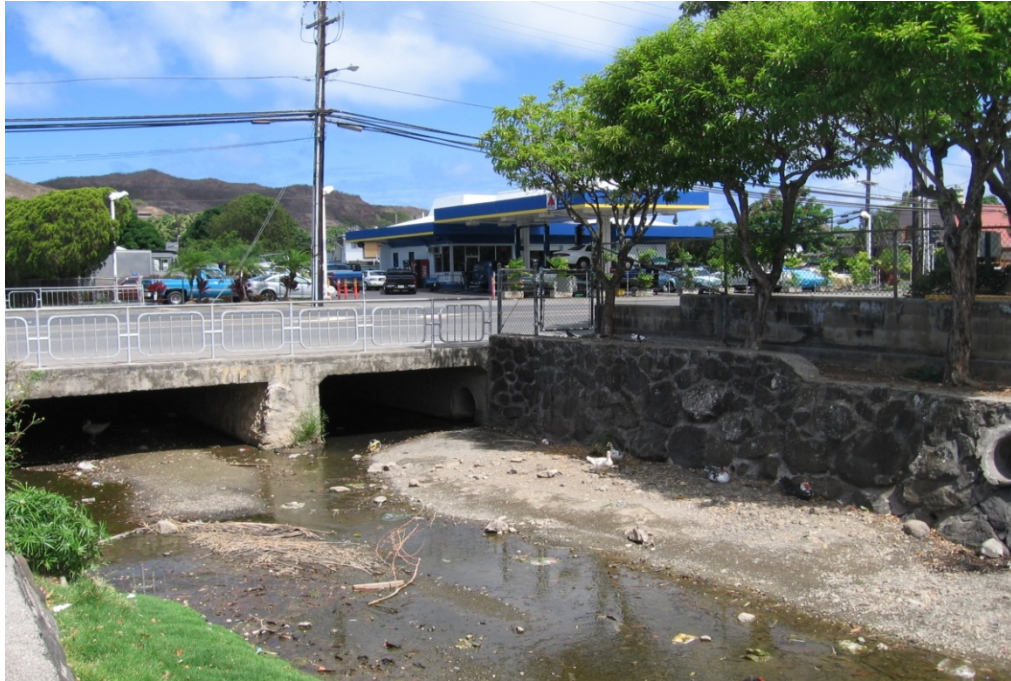
Photo 1-28 Hele Drainage Channel and twin Keolu Drive box culverts. Note RCP coming in from Enchanted Lakes Shopping Center to the right (south).
