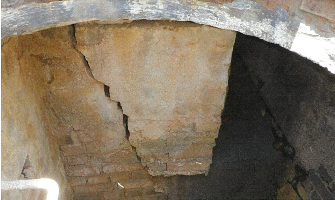
Photo 2 – CB #13 (Akahai Street) – Catch basin wall broken near wing. (Similar break in CB #14)
