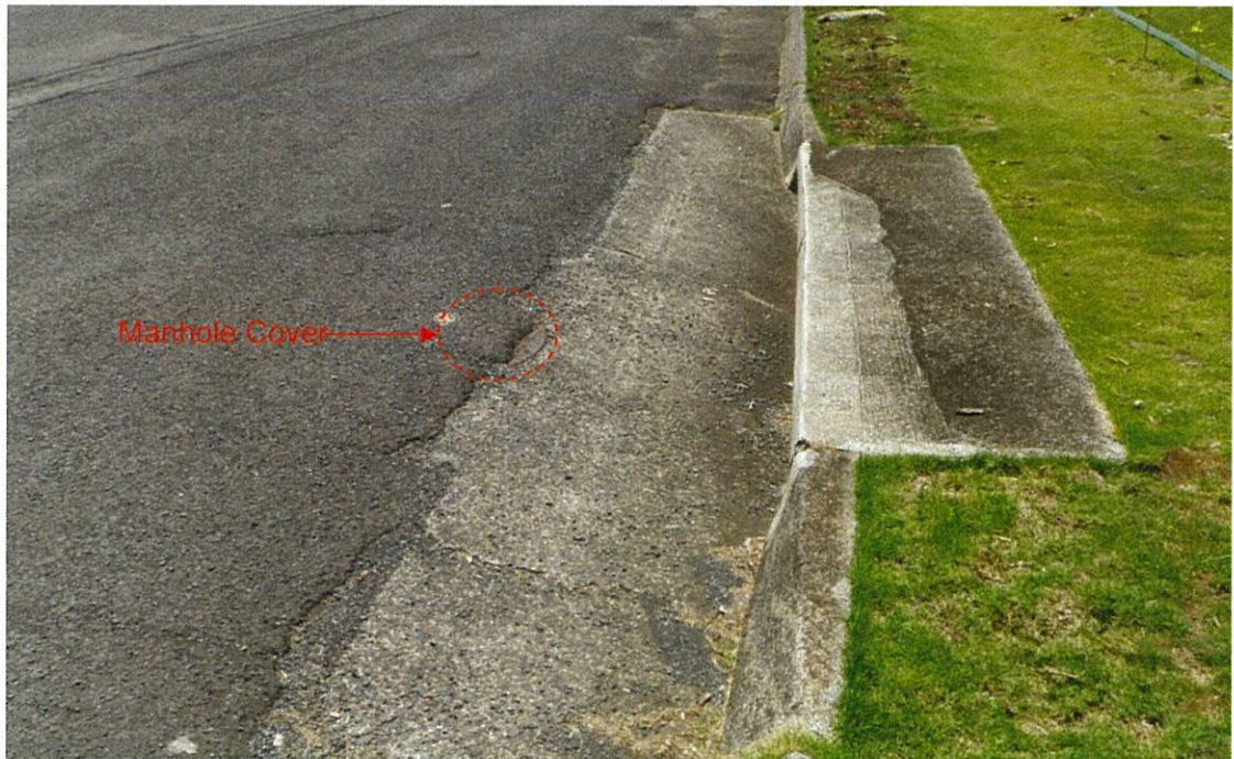
Photo 1 – CB #12 (Akaiki Street) – Manhole covered with asphalt.
