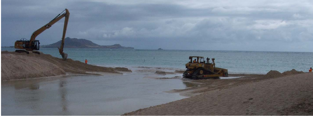
Figure 1.6 A long-reach excavator and bulldozer are typically used to conduct stream mouth openings.
