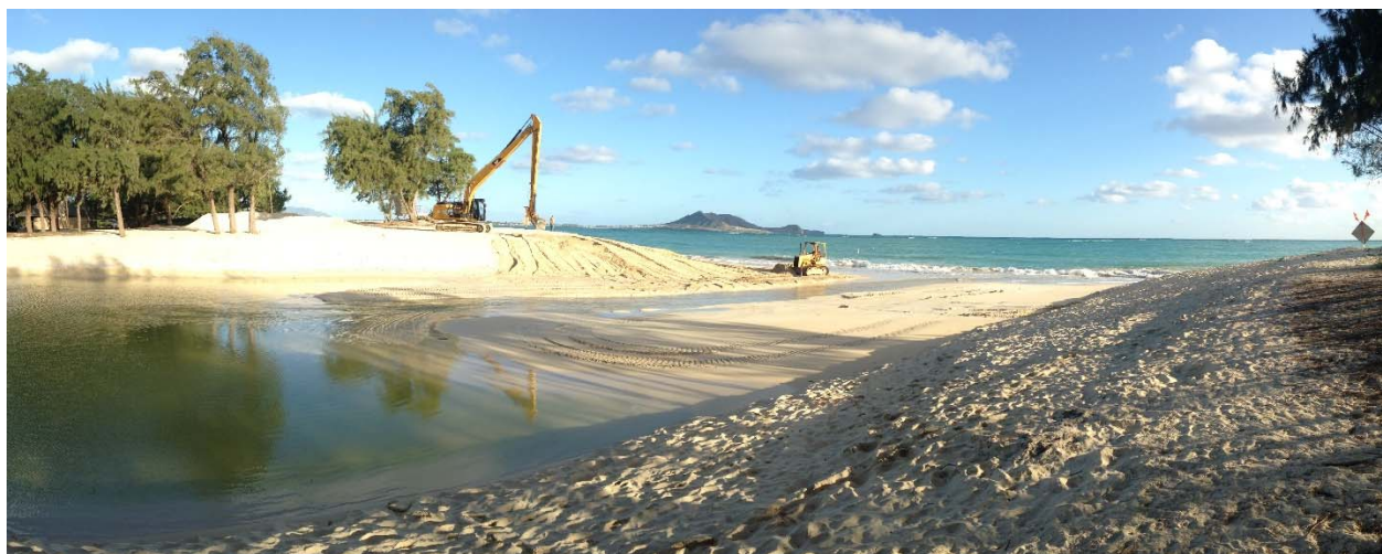
Figure 2.7 Opening the Kaelepulu Stream mouth at Kailua Beach using a small bull dozer and a long reach excavator. Beginning pile of excavated sand can be seen between trees behind the excavator.
