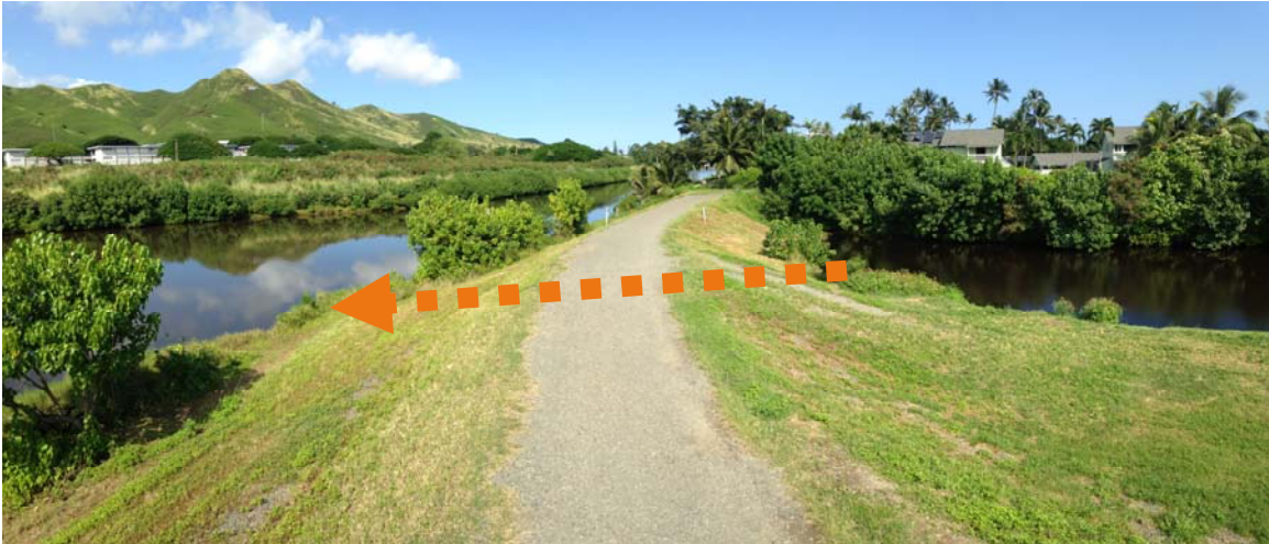
Figure 36. Levee where it separates Kawai Nui Stream (right) from Oneawa Canal (left).
