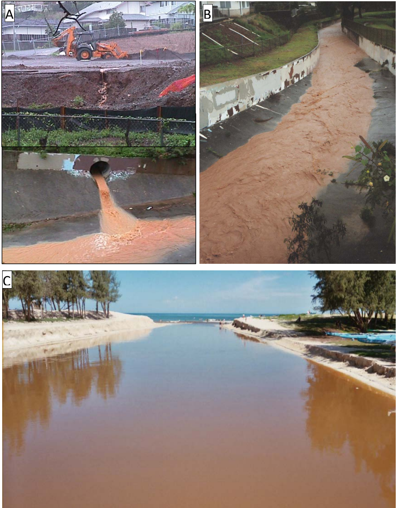
Figure 20 Construction activities (A) have the greatest impact upon delivery of sediment and nutrient turbidity to the pond (B) and into the ocean (C) when the stream mouth is open.
