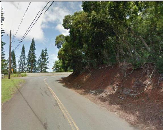
Unprotected Bare Road Cuts – the Old Kalanianaʻole Hwy was cut into the slopes of the hills. Most of the road cuts are bare, with vegetation roots exposed. The eroded material accumulated on the shoulder
